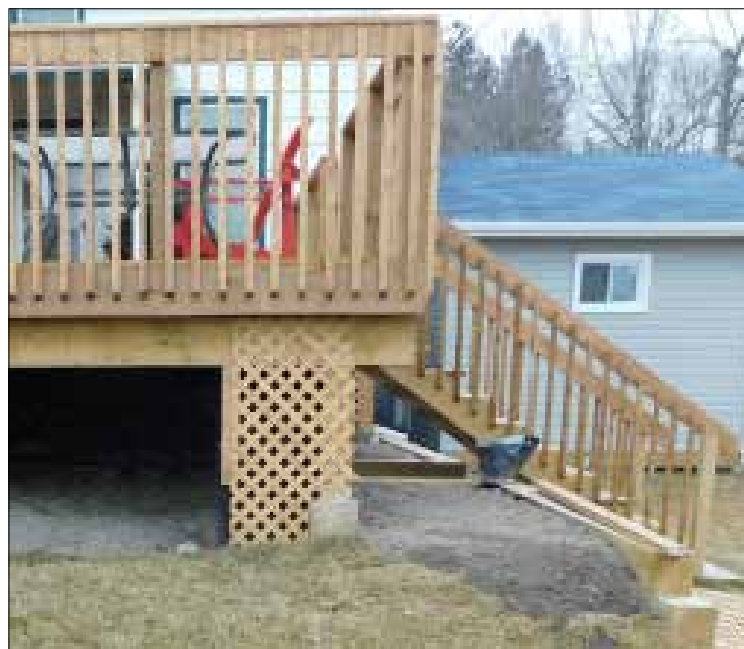
Restore property features including decks, structures, fences and landscaping to building code specifications.
