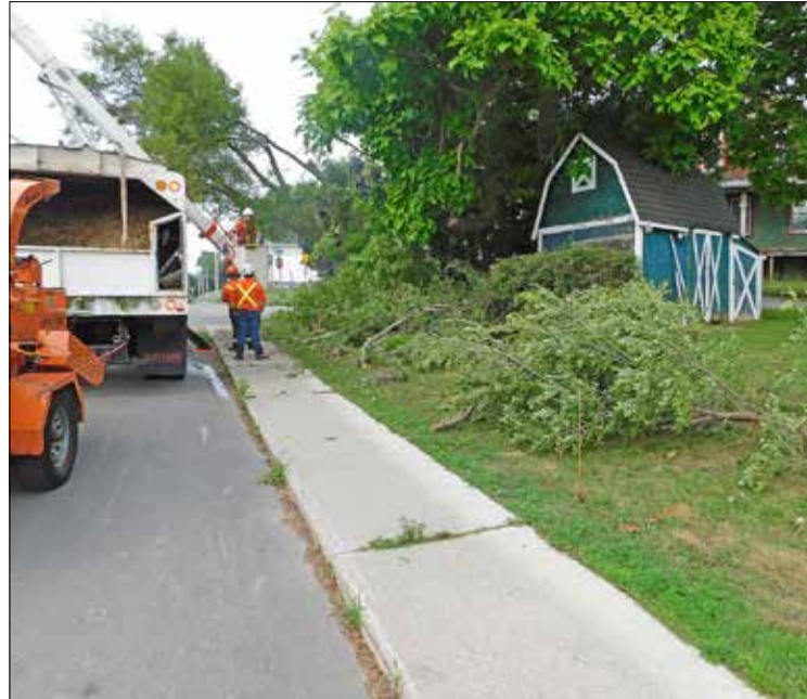
Remove trees, shrubs, impacted structures, store property owner items to facilitate cleanup.
